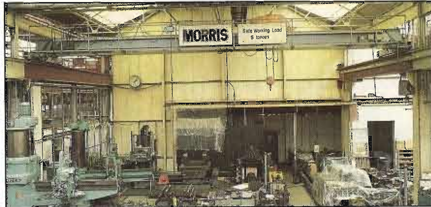
Morris 5 Tonne Twin Girder Electric Overhead Travelling Crane, 42' Span
