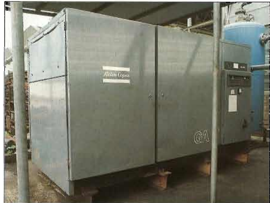
Atlas Copco 'GA808' Rotary Screw Air Compressor
