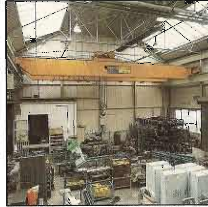
Morris 25 Ton Twin Box Girder Electric Overhead Travelling Crane, 42' Span
