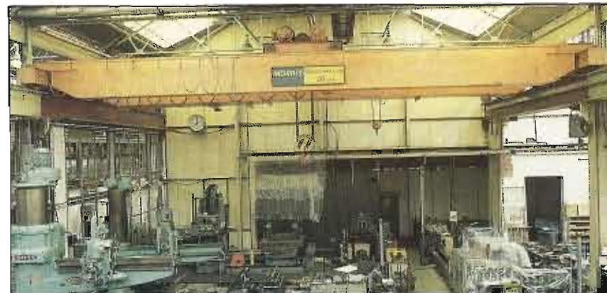
Morris 20 Ton Twin Girder Electric Overhead Travelling Crane, 42' Span
